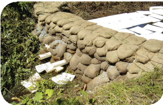
Inverted weir dam allows clean water to flow from the bottom so floating oil is blocked at the surface
