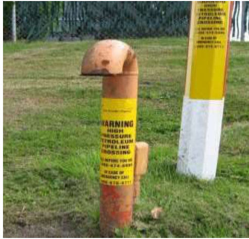
Casing Vent Marker
