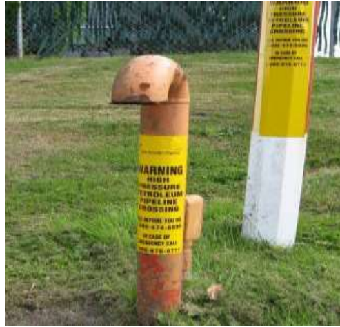
Casing Vent Marker
