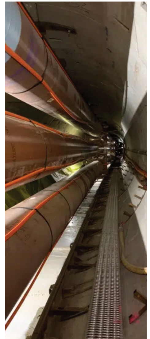
Top and below: State-of-the-art fibre optic system deployed on pipeline for the Trans Mountain Expansion Project
